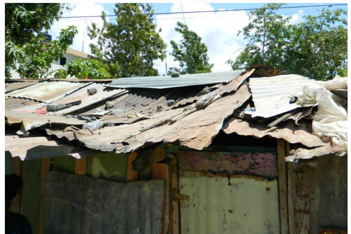
The roof in very bad conditions – March 2015
